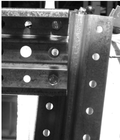
Fig. 16: Portal beam to upright connection deformation during phase 3
