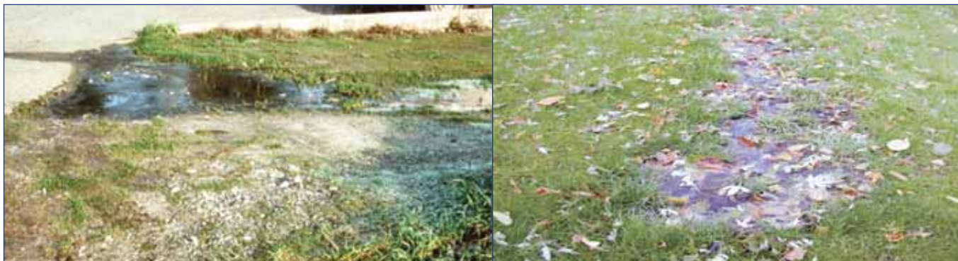
Figure 6. Examples of surface surcharging of septic tank effluent due to hydraulically failing septic absorption system.
