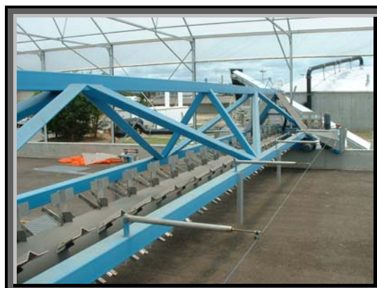
Figure 2. Mechanical sludge turner.
