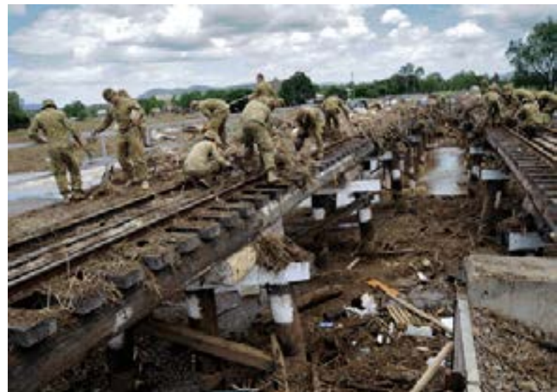
Soldiers from 8th/9th Battalion, Royal Australian Regiment (RAR), and engineers from the 2nd Combat Engineer Regiment (CER), based at Gallipoli Barracks in Enoggera, clear the train line that runs through Grantham following the 2011 Queensland floods. (Defence Image Gallery | Petty Officer Damian Pawlenko)
