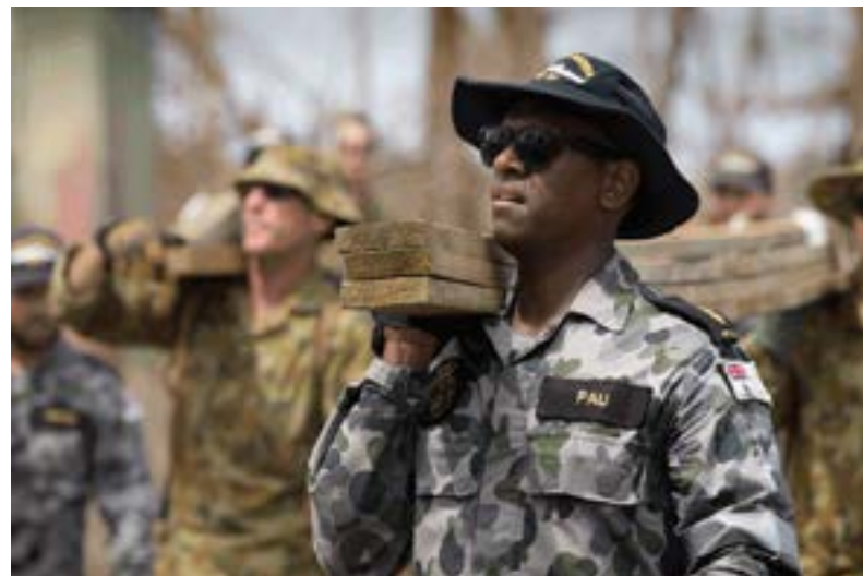
Royal Australian Navy sailor Able Seaman Boatswains Mate from HMAS Canberra, helps carry timber that will be used to repair schools on Taveuni Island on the Eastern side of Vanua Levu, Fiji's second largest island as part of Operation FIJI ASSIST 2016. (Defence Image Gallery | LSIS Helen Frank)
