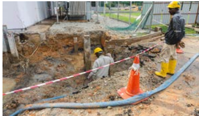
Foreign workers do the installation of cement formwork frames at a construction site. (Shutterstock | Lemau Studio)
