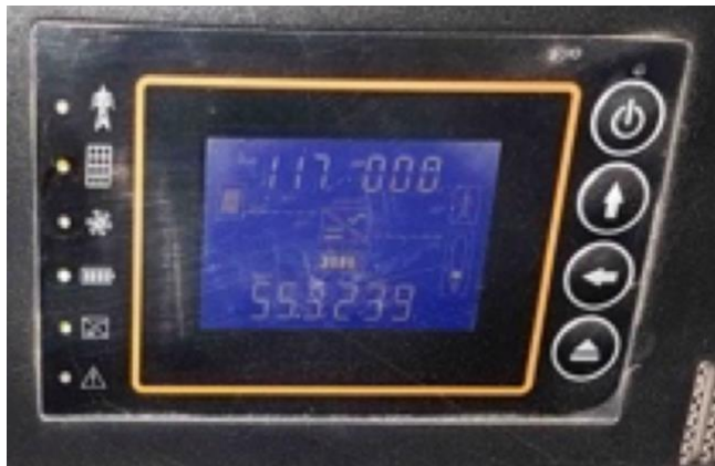
Image of an LCD display from one of the mini power systems installed
