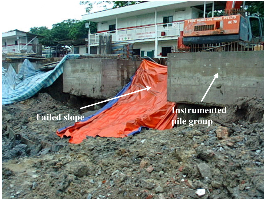
Fig. 6. Slope failure that unexpectedly occurred next to the instrumented pile group (Day 0)
