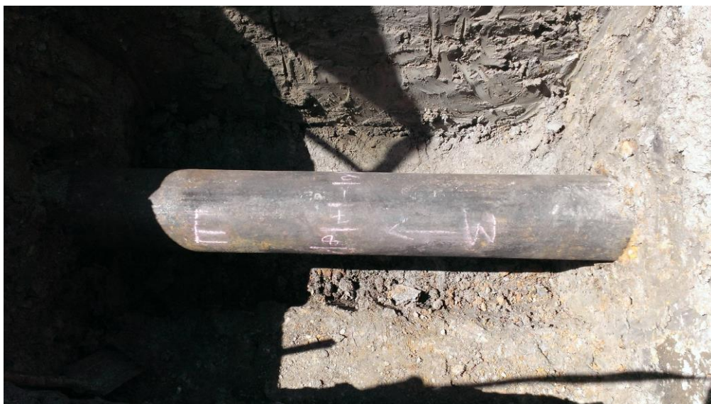
Figure 1: Photo of excavated pipe
