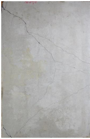
(g) Wall WS2a tension face
