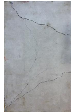
(e) Wall WS1c tension face
