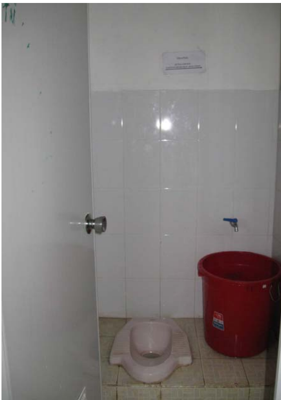
Figure 7.2. Female toilet in school A
